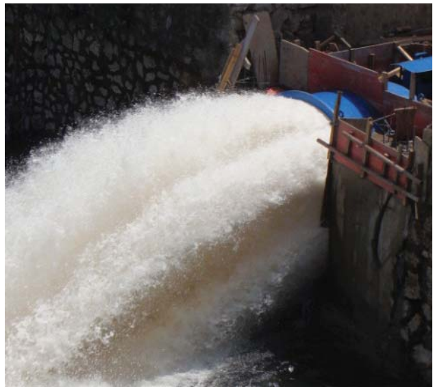
Free discharge of continuous flow
